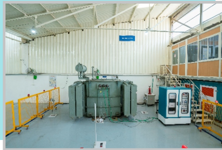
Measurement of short-circuit impedance & Load loss at 50% & 100% load
