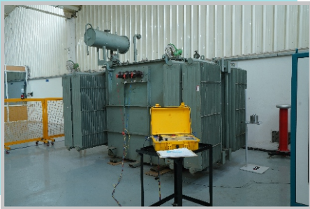
Measurement of voltage ratio & check of phase displacement / voltage vector relationship
