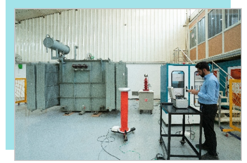
Separate source voltage with stands test
